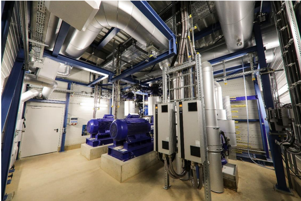
Block-Type Thermal Power Station in Cologne Merheim ©RheinEnergie AG
