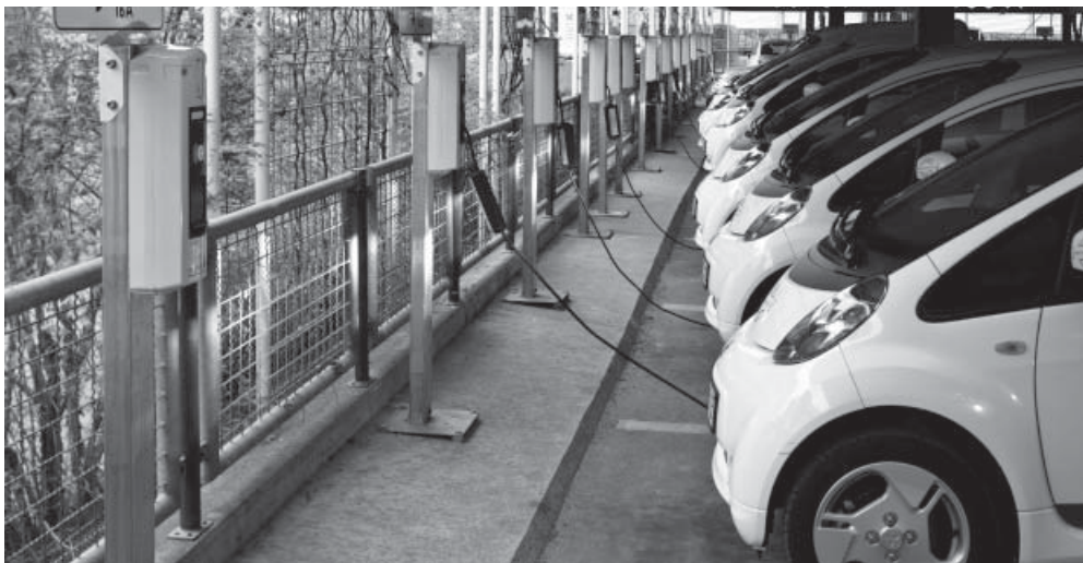
Up to 30 electric vehicles at a time can recharge in Fraunhofer IAO's parking garage. (© Victor S. Brigola/Fraunhofer IAO) | Picture in color and printing quality: www.fraunhofer.de/press
